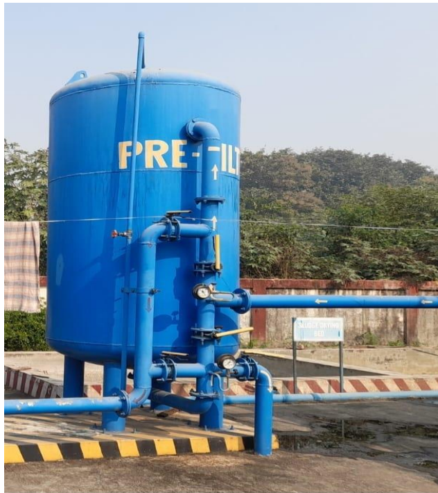
Fig. 7. Primary filtration process (Source-Northern Eastern Railway Gorakhpur)
