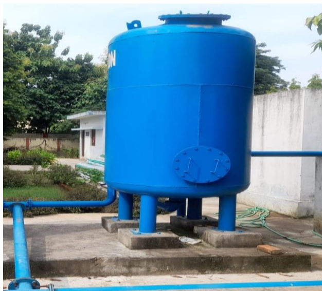
Fig. 8. Primary filtration process (Source-Northern Eastern Railway Gorakhpur)
