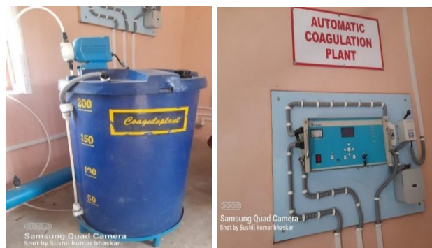
Fig.1& 2. Coagulation Process (Source-Northern Eastern Railway Gorakhpur)
